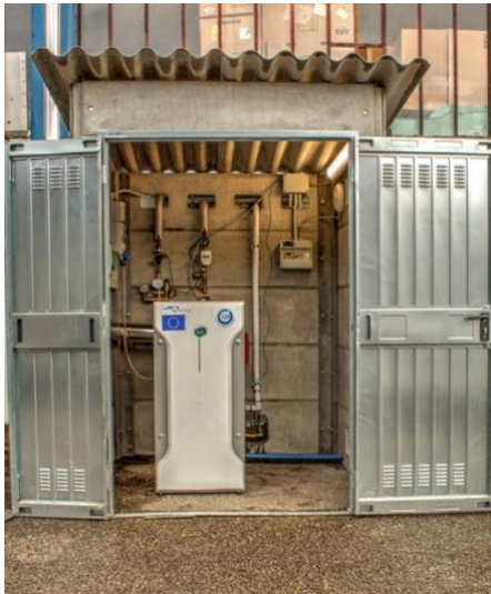
New Electric Store (Electric Materials Store)
